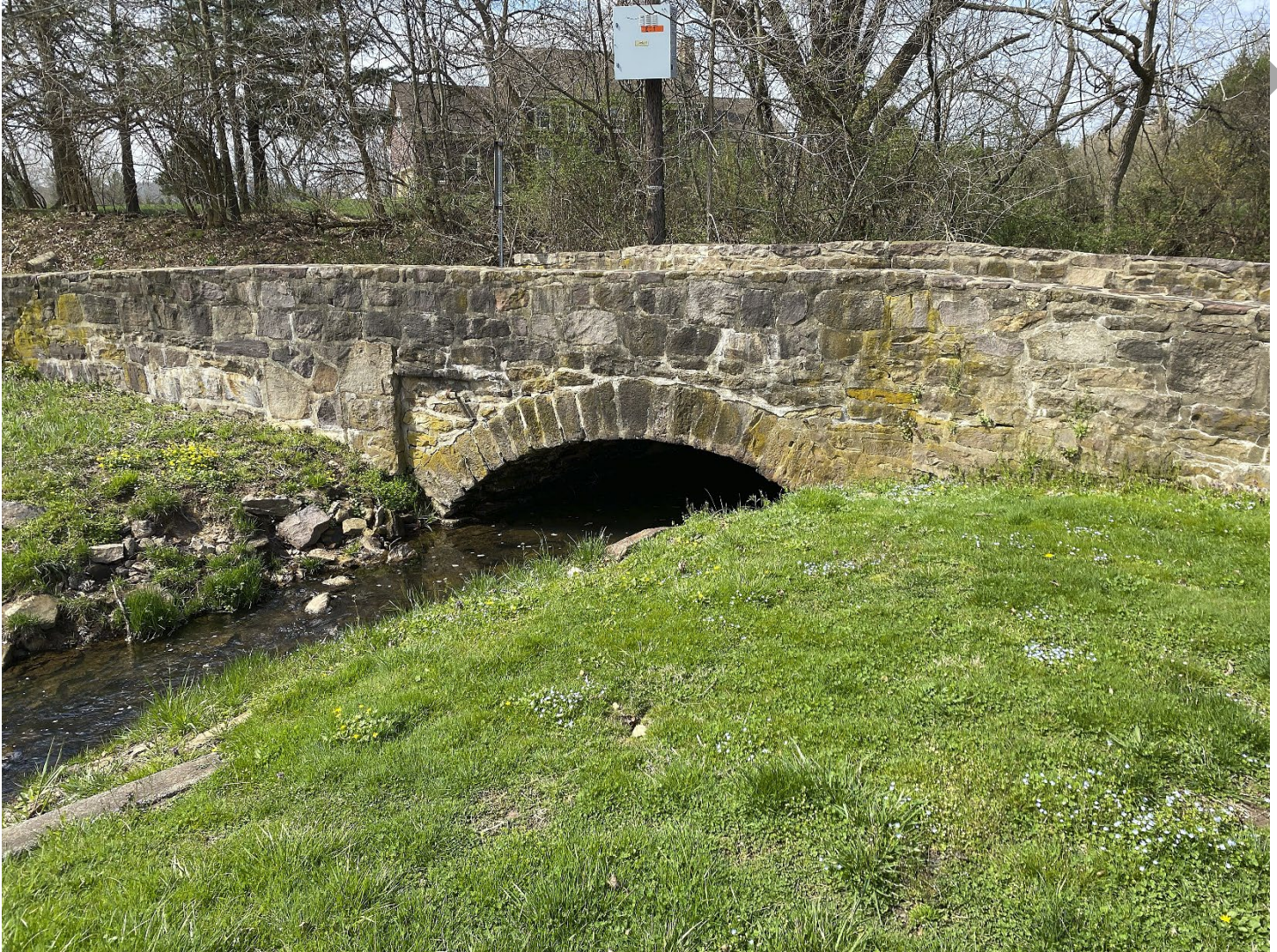
Photo 6: East (downstream) side of the bridge showing the low segmental arch, view facing northwest
