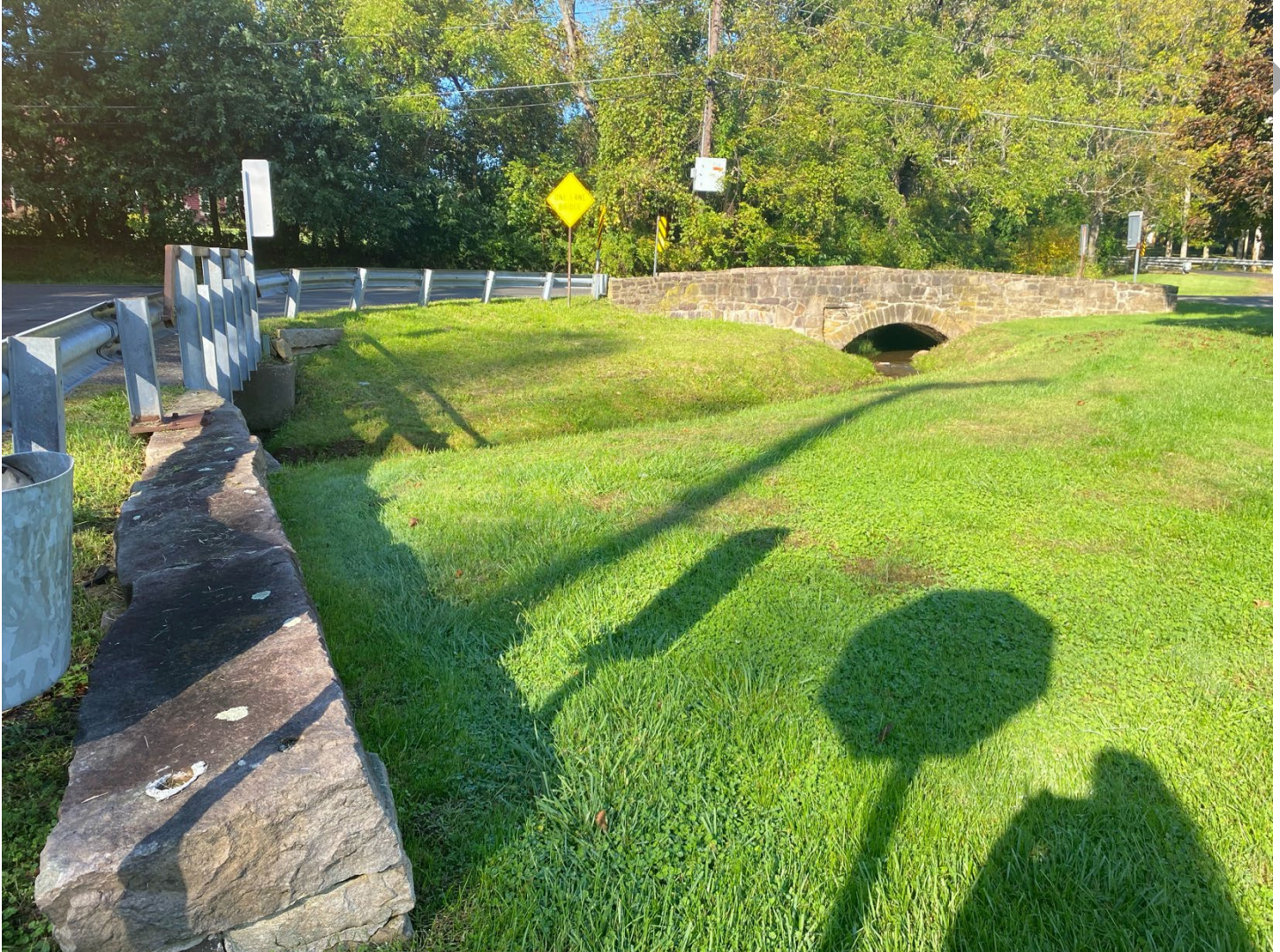
Photo 2: East (downstream) side of the bridge, View facing west from the adjacent bridge on Dunkard Church Road
