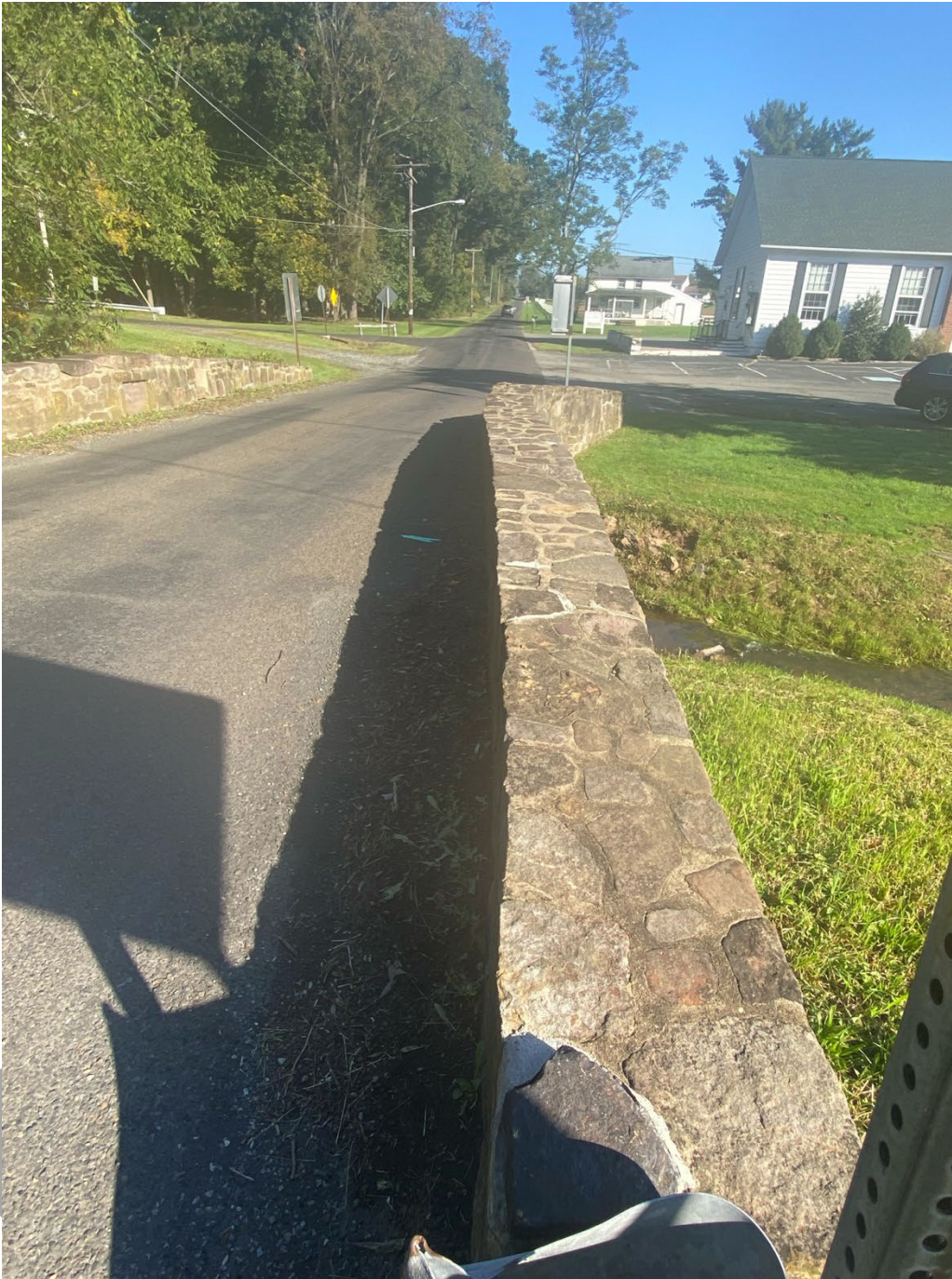
Photo 9: East (downstream) wingwalls and parapet, view facing north showing the absence of capstones.
