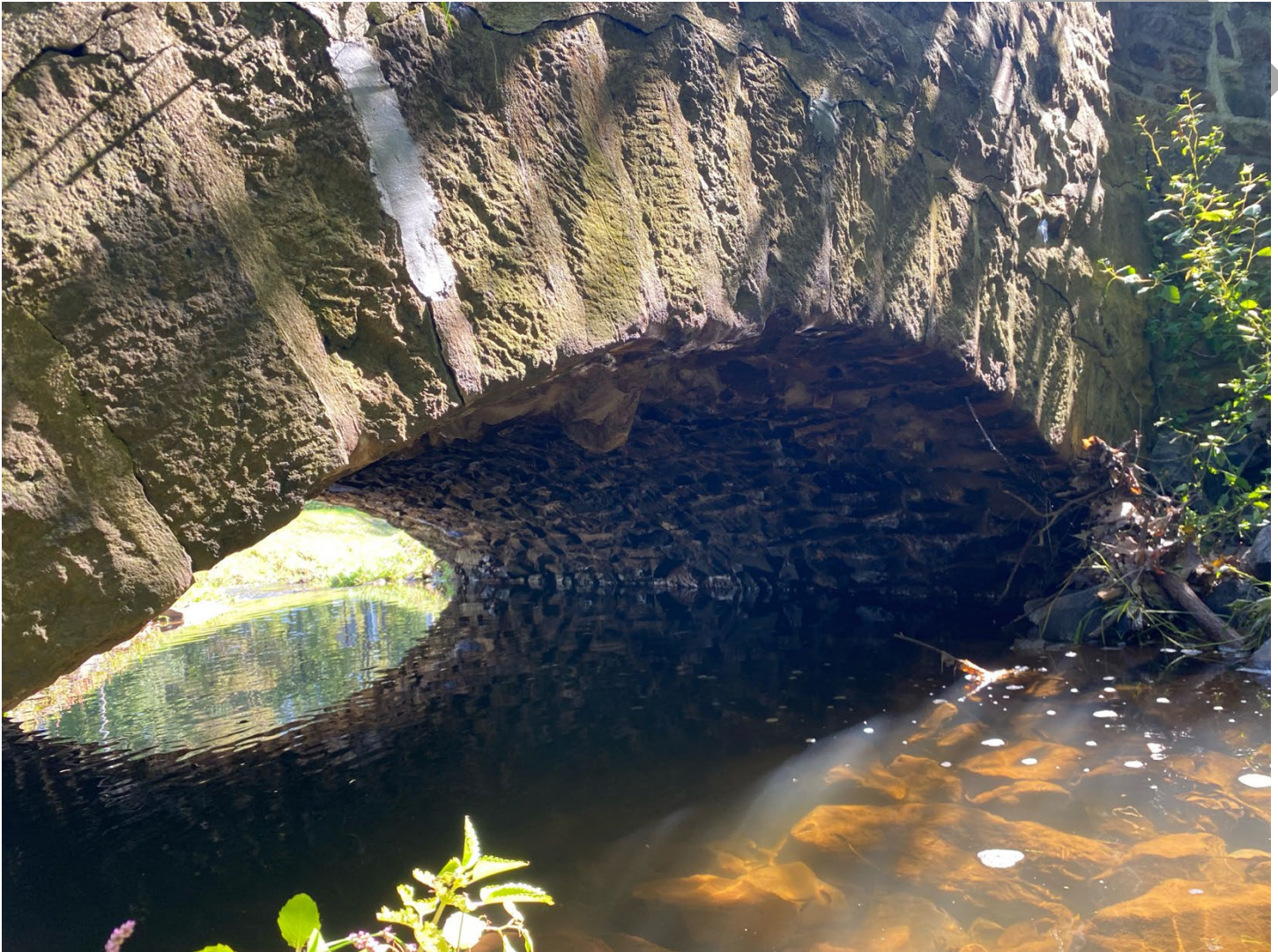
Photo 7: West (upstream) side of the bridge, showing the low segmental arch, view facing southeast
