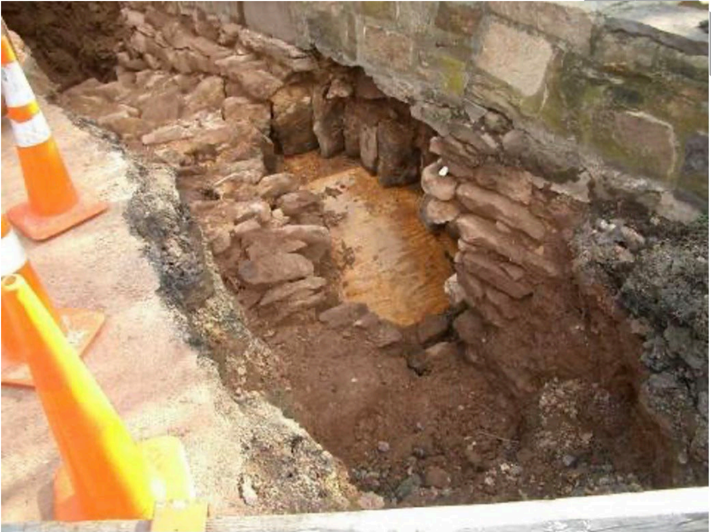
Illustration 9: Collapsed section of the barrel vault after removal of the road surface. Complements of Chuck Taylor 2009.
