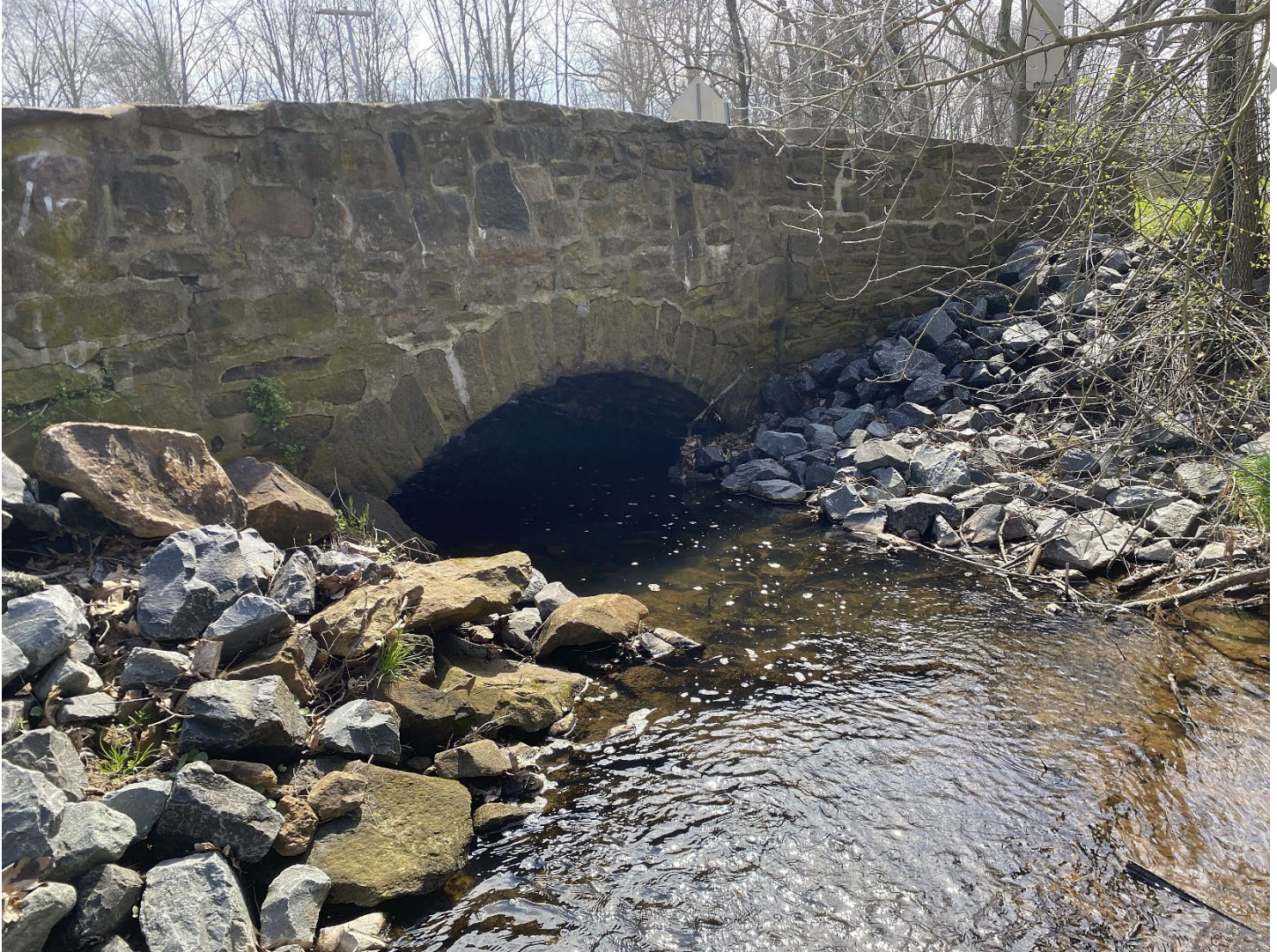
Photo 4: West (upstream) side of the bridge, view facing southeast from the stream
